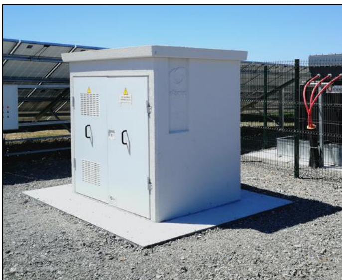
Plate 4-7. Outdoor cabin switchgear
