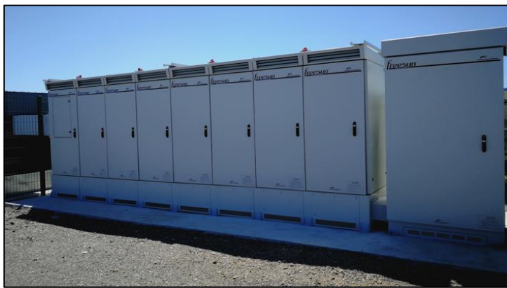
Plate 4-4. Typical outdoor centralised inverter
